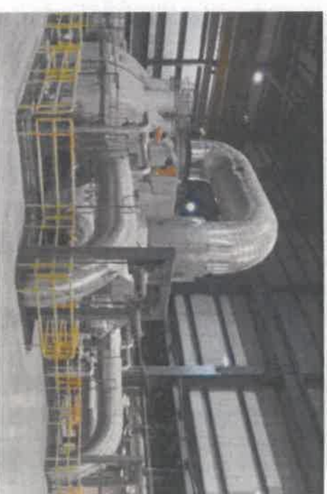
Photo from inside the AMP Fremont Energy Center (AFEC). AFEC is a natural gas, combined cycle facility that has a capacity of 512 MW (unfired) and includes duct firing that allows an additional 163 MW of generation during peak demand periods. It provides power for 86 Member communities that participate in the AFEC project, which includes Richlands.
